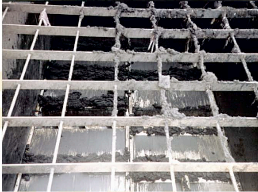
Truck reception bunker in pit showing safety grid
